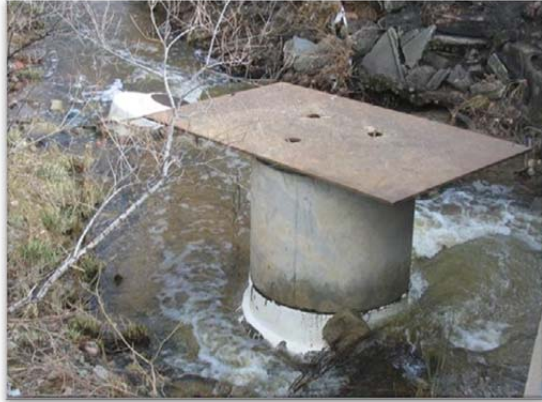
Above: A sheet of metal acts as a temporary cover on a sewer manhole in Miller Creek that overflowed during a storm.
